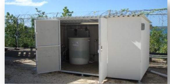
MIOX on-site generator in portable building
