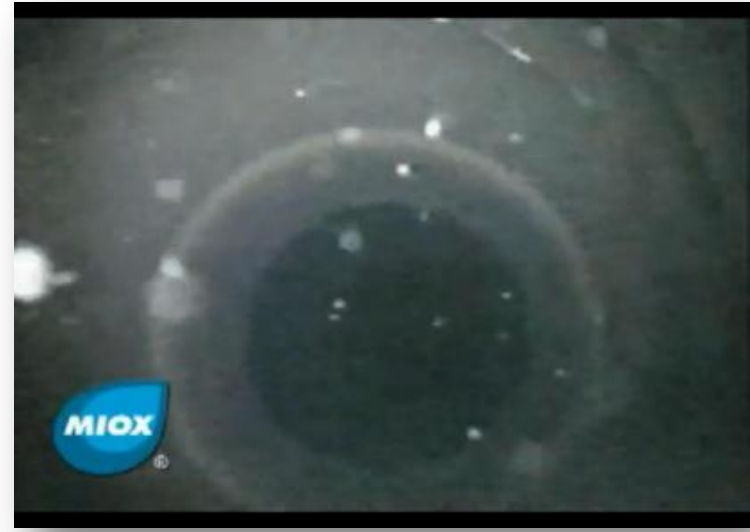
Filter recirculation pipe 22 days after MOS
