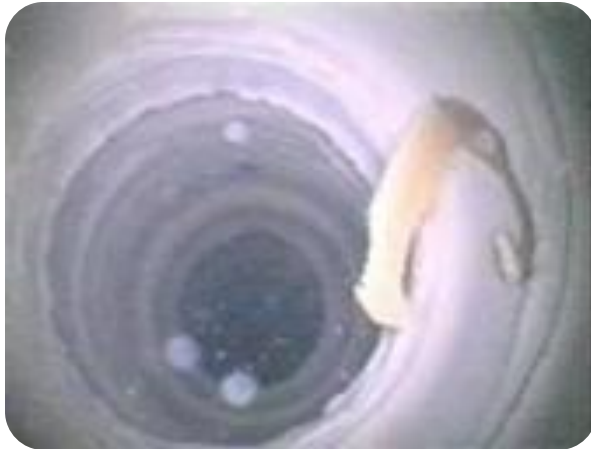
Filter recirculation pipe with sodium hypo
