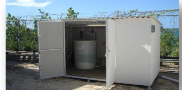
MIOX on-site generator in portable building
