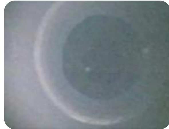
Filter recirculation pipe 22 days after mixed oxidant solution
