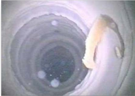
Filter recirculation pipe with sodium hypo
