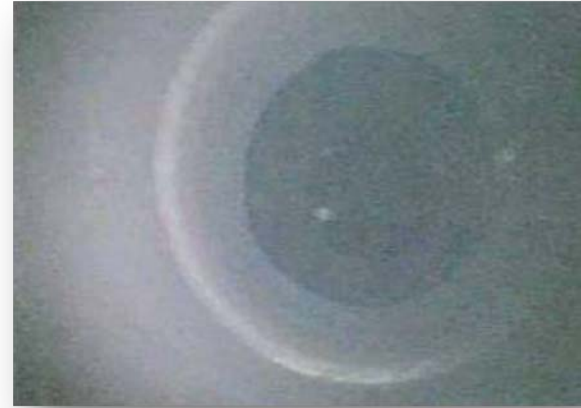
Filter recirculation pipe 22 days after mixed oxidants
